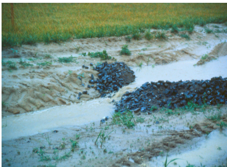
Check dam (Source: Auckland Council)
