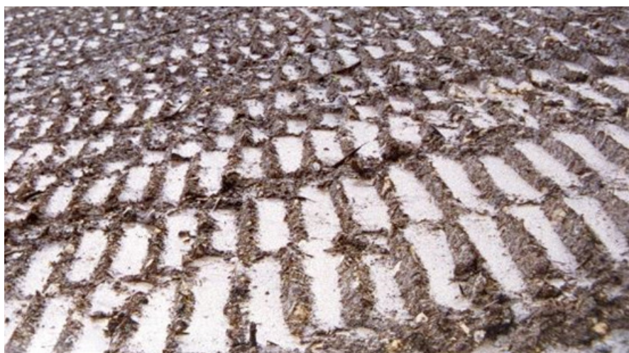
Surface roughening of a slope. Note that the hollows act as 'micro' sediment traps
