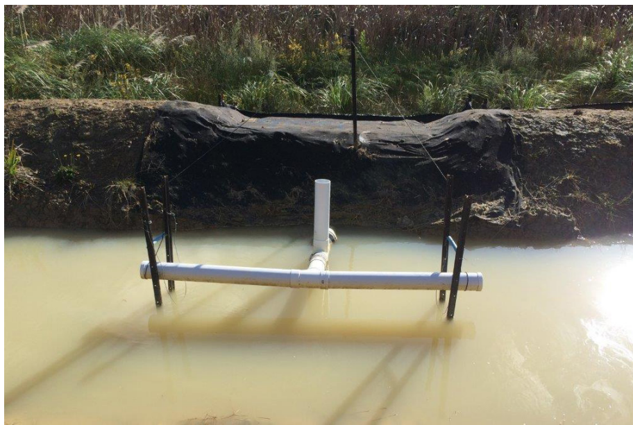
Close up of decanting earth bund system (Source: SouthernSkies)
