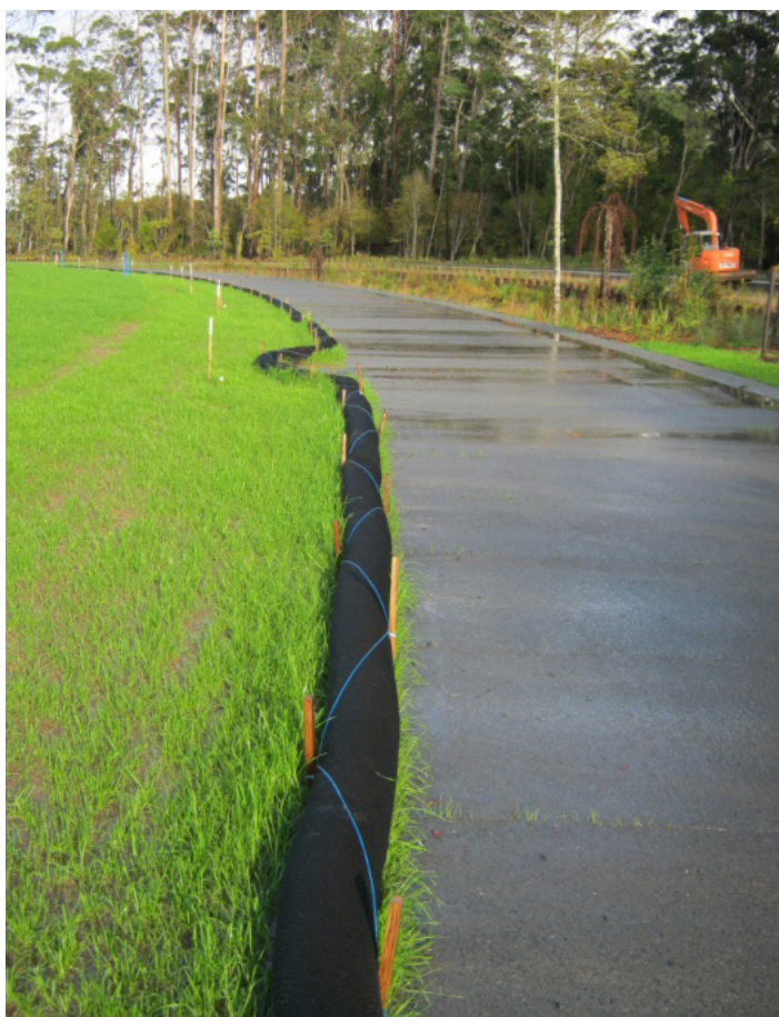
Silt sock used to provide control during final landscaping works (Source: Erosion Control Ltd)
