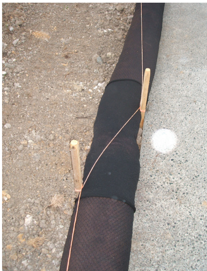
Silt sock joined using a sleeve and pegged and secured using bailing twine with 1 m overlapping joint (Source: Erosion Control Ltd)
