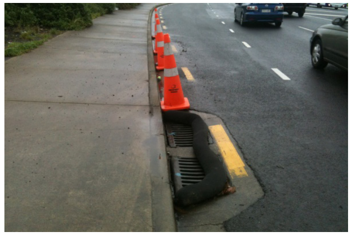
Installation of a silt sock to provide some protection to the catchpit
