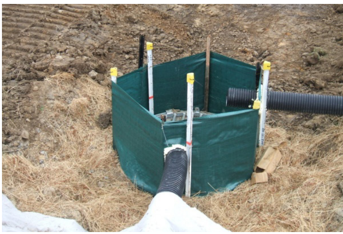
Good use of a silt fence installed to protect a new stormwater catchpit where impounded water will not create a flooding hazard
